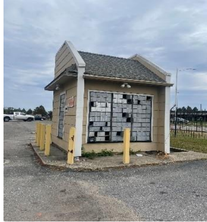
Figure 12: Image of a mailbox taken by Jane Place staff at an apartment complex from where many T.E.E.N.S. postcards have been returned. Broken mailboxes are left unlocked and open, with mail scattered around the parking lot.
